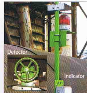
Conveyor Starting Indicator
