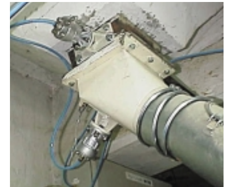
Flour mill plant Chute
