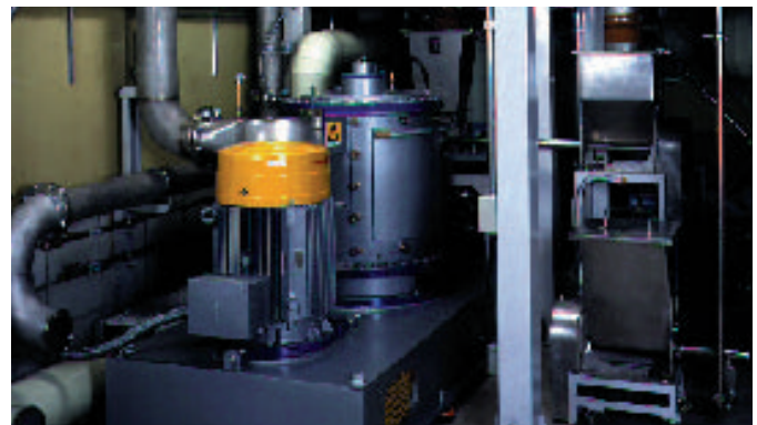
SR-75 at use in a Toner Plant.
