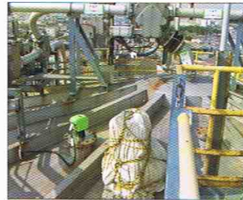
Pulse radar level meter at chemical powder silo
