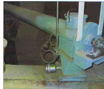
Microwave Flow Switch for screw feeder
