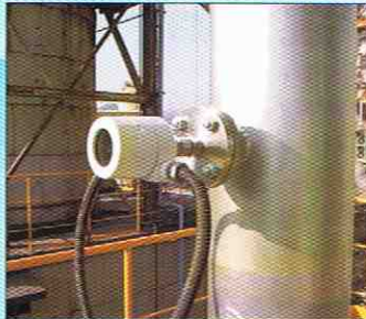
Dust Monitor (compact type) at bag filter outlet
